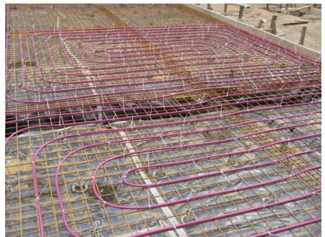
A hydronic underfloor heating installation
